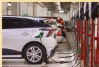
EV CHARGING POINT
